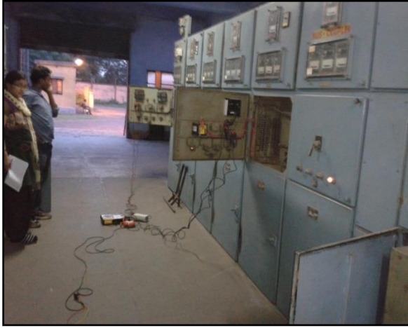
Students measuring power in a Substation
