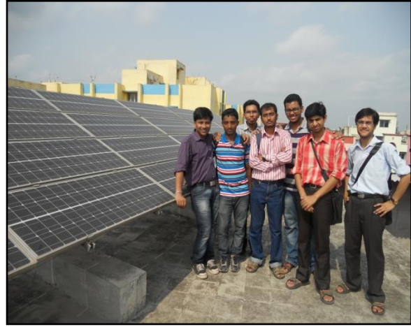
Field visit at 4\text{kW}_p Solar Roof top power plant
